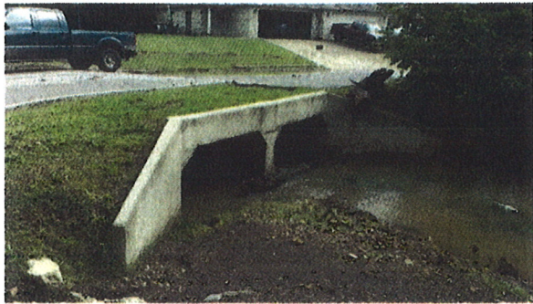
Figure 1 Drainage Creek Under Rainsong - Day After Flooding
