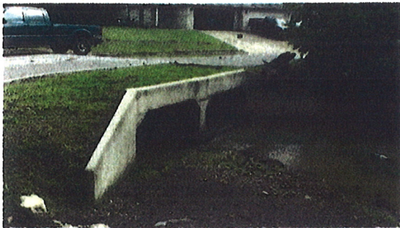
Figure 1 Drainage Creek Under Rainsong - Day After Flooding
